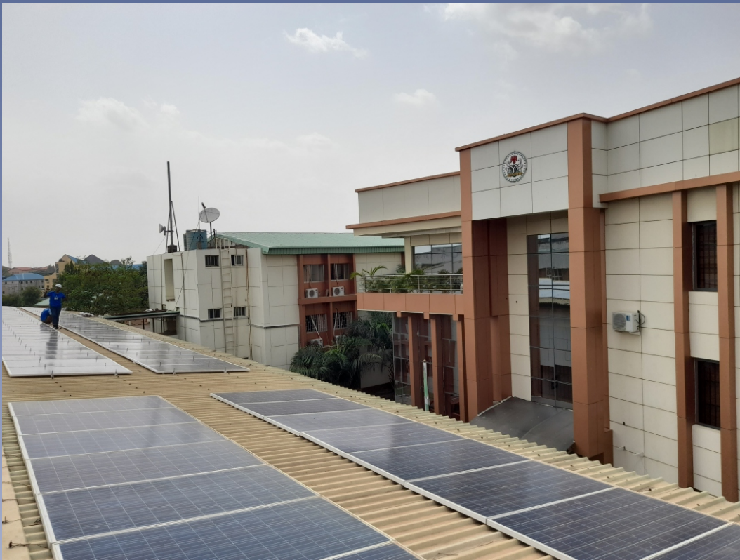
Installation Of 40kw Solar Off-grid System At Federal Ministry Of Interior Headquarters, Abuja
