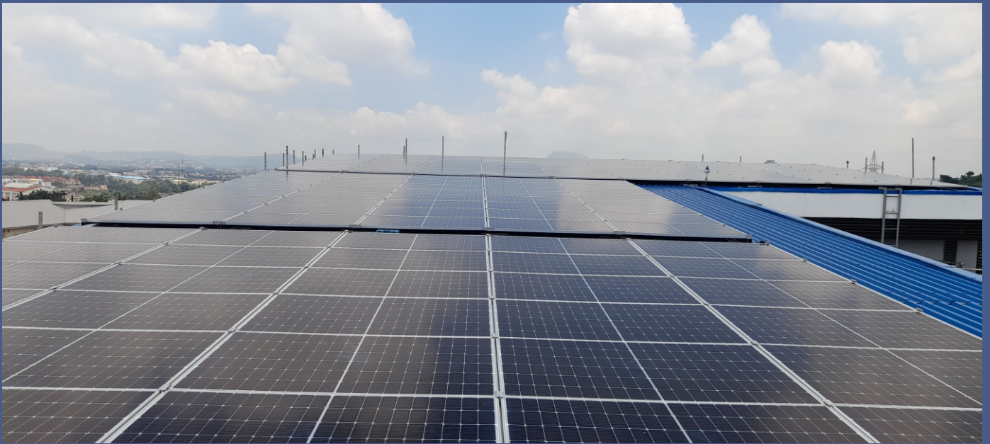
152KWP Solar Installed Capacity at JRB Headquarters
